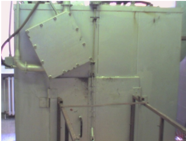
Figure 3. Industrial furnace – door
