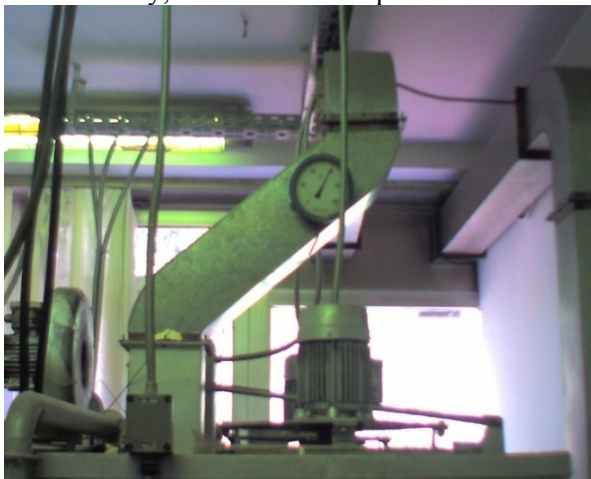
Figure 5. Industrial furnace-ventilation system
