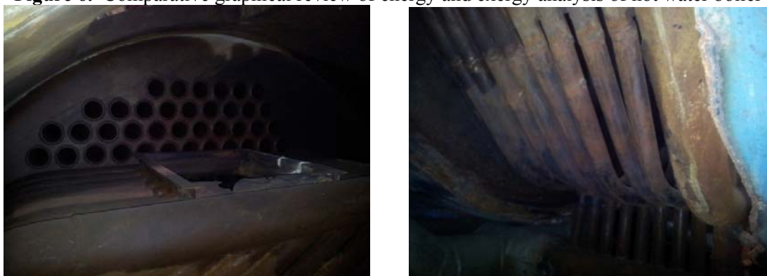
Figure 7. Damaged water-cooled pipes of the diverting chamber of the hot water boiler (left and right)
