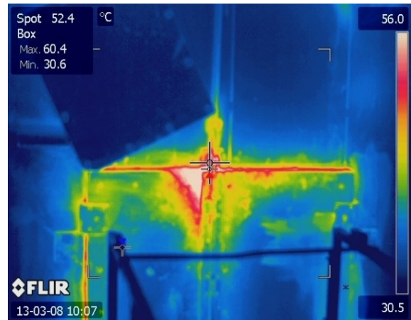
Figure 4. Thermography examination of the door of industrial furnace
