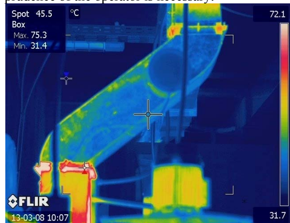
Figure 6. Thermography examination of ventilation system of industrial furnace
