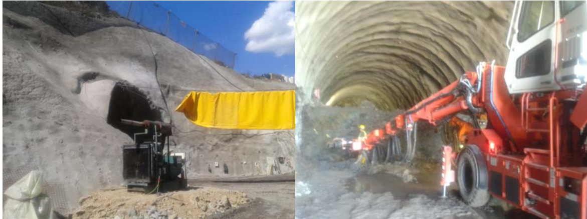
Figure 1. Tunnels T1 (T2) as primary sources of air pollution on site Tunnels are drilled with multiple methods of blasting of rocky material (fig. 2 and 2b) (strictly controlled explosions) and drilling with machinery (such as fig. 1b).
