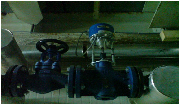
Figure 3. Electrical regulating steam valve
