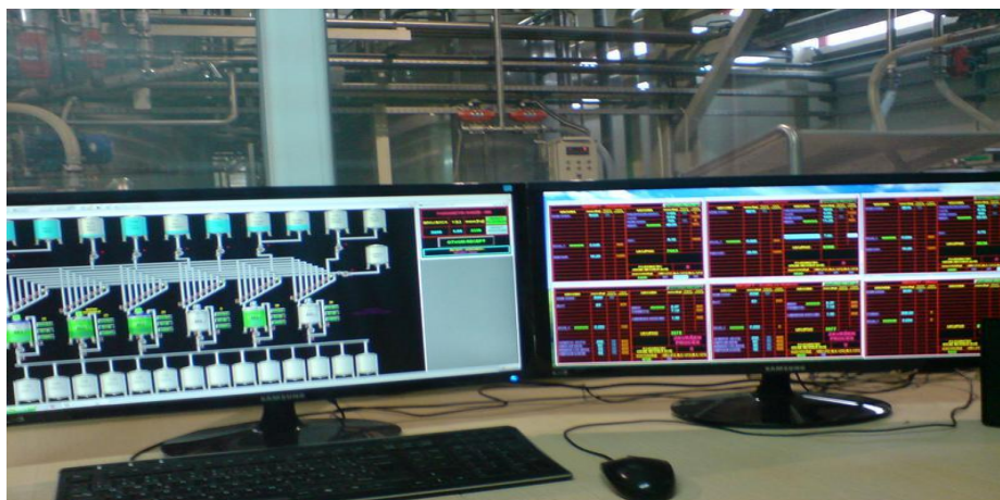
Figure 6. Command room from where the process is monitored
